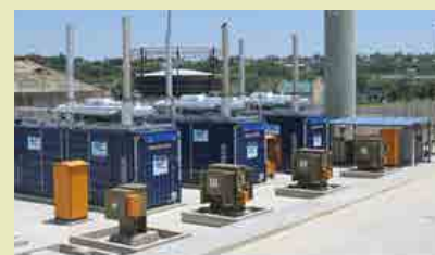
Figure 2: Generators at Northern Works
