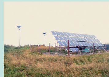
Figure 3: Vandalised PV panels at Hluleka Nature Reserve
