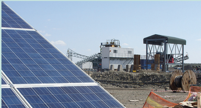
Figure 4: PV installation at Thabazimbi Mine
